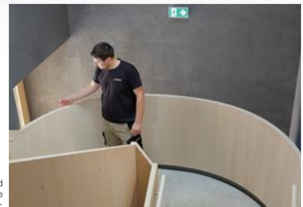
A BARTH vacuum press was used to manufacture the handrail in the staircase of the company Rüscher.
